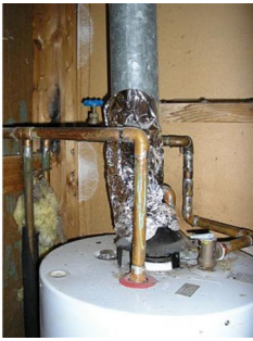
27-1. Water Heater(s) SAMPLE PICTURES
