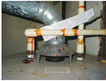
27-2. Water Heater(s) SAMPLE PICTURES
